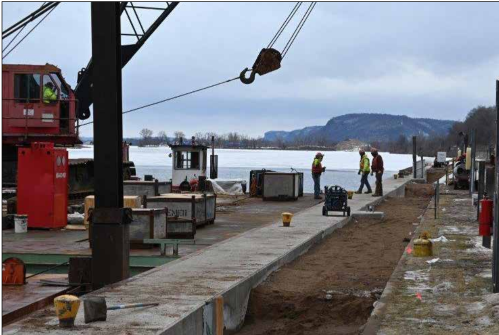
Work continues on the tow rails at Lock and Dam 4 in Alma, Wisconsin, Feb. 9. USACE photo by Patrick Moes
