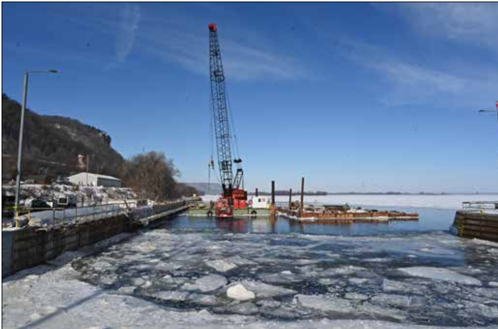
Construction progresses on the Lock and Dam 7 tow rails in La Crescent, Minnesota, Feb. 8. USACE photo by Patrick Moes
