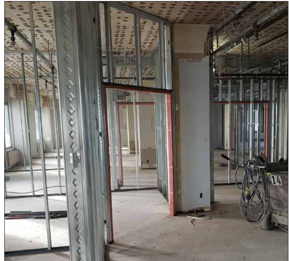
Building progress continues at the First National Bank building in St. Paul, Minnesota. USACE courtesy photo
